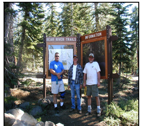
The Motherlode Rockcrawlers install trailhead signs on the Amador Ranger District, Eldorado National Forest.
